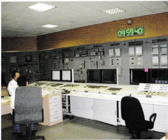
IBR-2M control room
