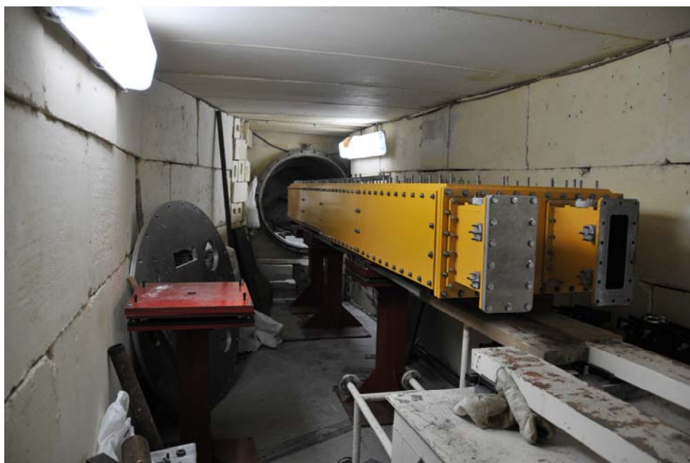
Fig. 10. The head part of the mirror vacuum neutron guide installed on beam 6 of the IBR-2 reactor within the framework of realization of the project of construction of the DN-6 diffractometer for microsample investigations.
